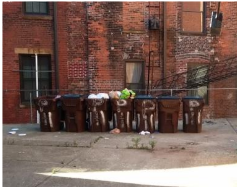
Garbage management neglected. Overflowing receptacles are the norm for many buildings, not safe or sanitary, attracts vermin.
