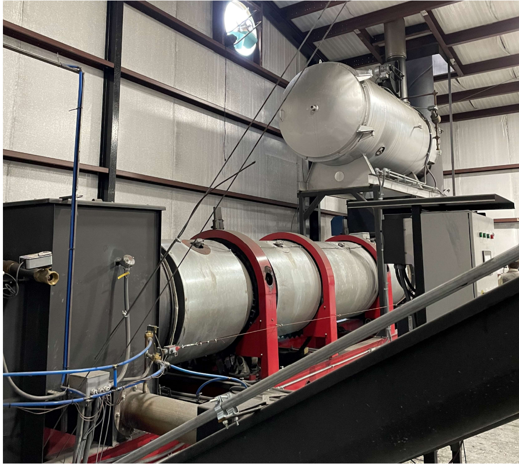
Boiler on top of Pyrolysis Unit
