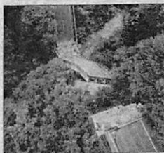
A bridge collapsed in Ichinoseki, Japan, when a magnitude 7.2 earthquake ripped across the northern part of the country on June 14, killing at least three people.
