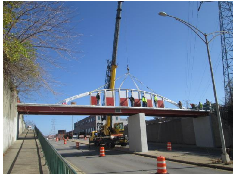
Installation of the prefabricated arch on the Madison Road Pedestrian overpass east of IORY
