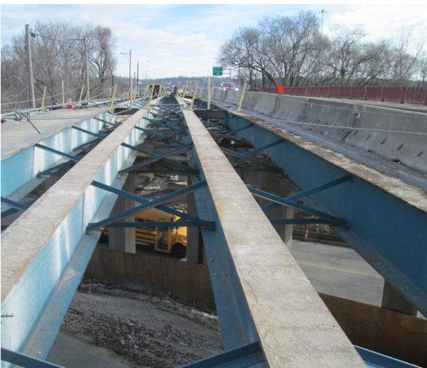
Ongoing construction at the Galbraith Rd Bridge over Anthony Wayne and railroads.
