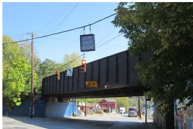
Low clearance automated warning system at railroad overpass over Madison Rd near Kenwood.
