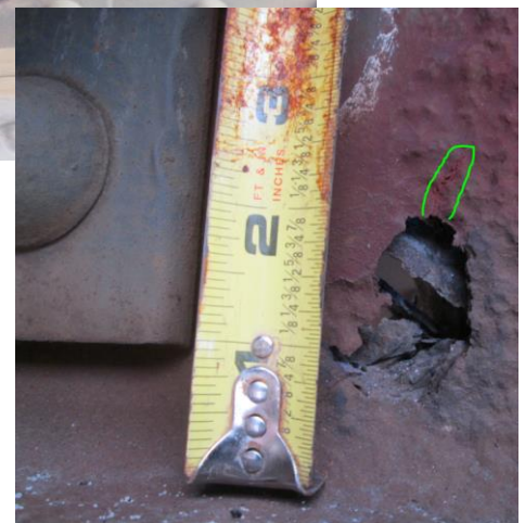
Sheared off bolts and corrosion holes at stringer to floorbeam connection on the 5 th Street Chessie overhead west of Linn Street
