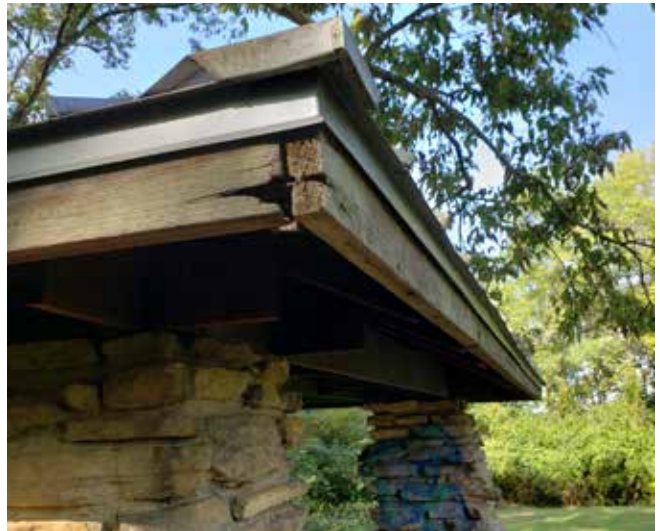
22. Mt. Echo shelter roof damage
