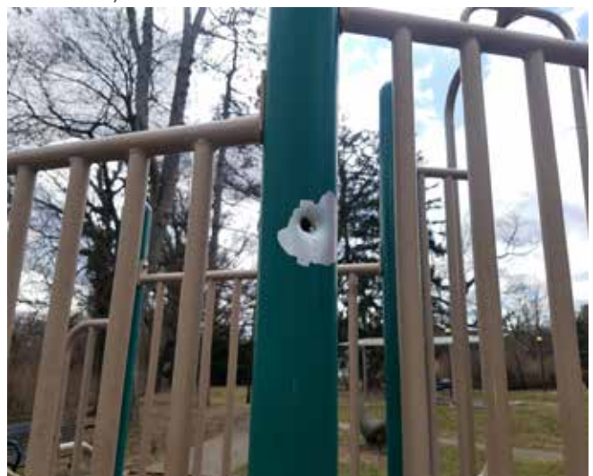
6. Stella Park damaged playground
