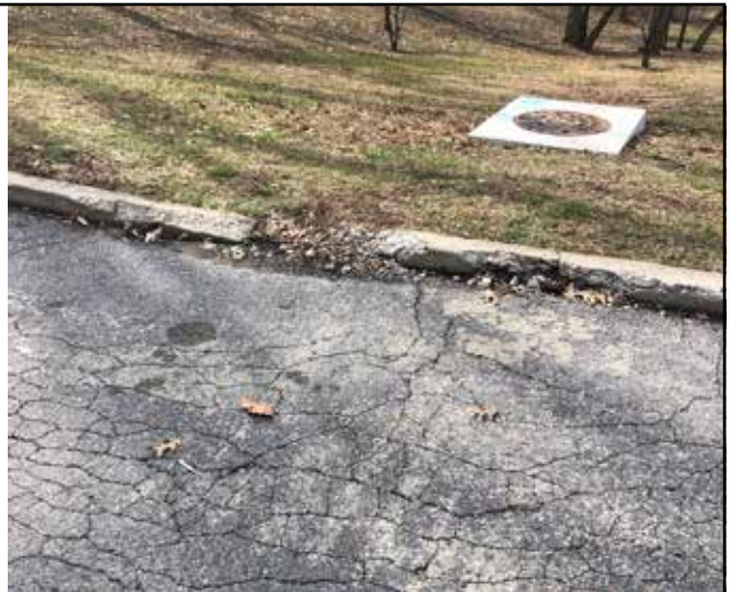
8. Eden Park damaged curb
