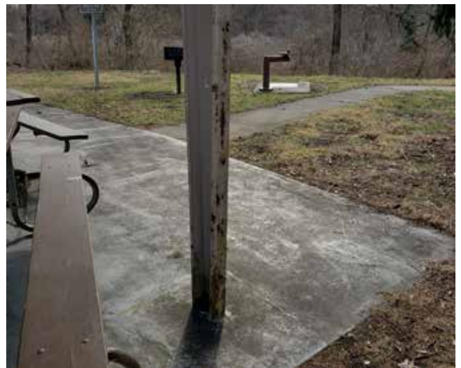
18. Stella Shelter rusting posts
