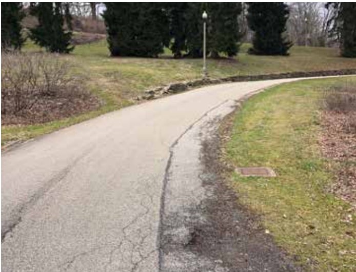
3. Alms Park deteriorating pavement
