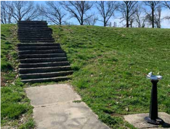
15. Mayfield steps with no handrails
