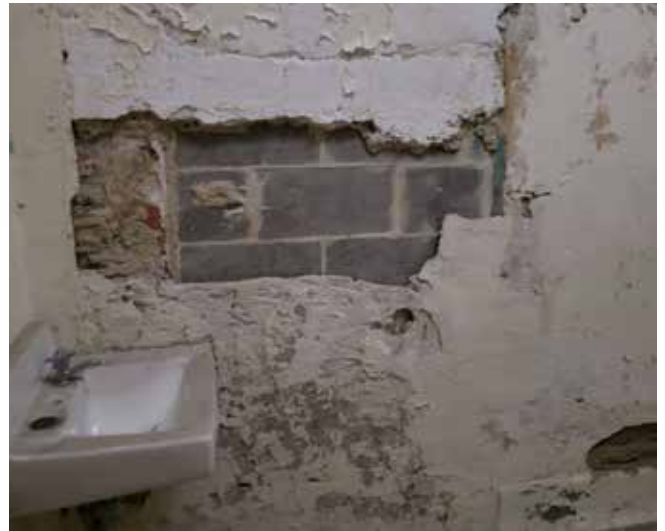
2. Inwood Pavilion decaying interior
