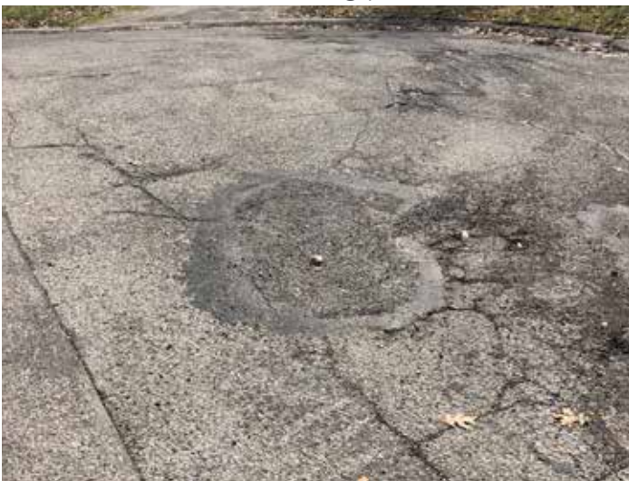
5. Mt. Echo poor pavement
