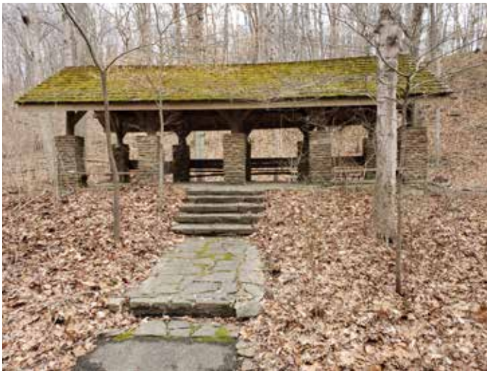
13. California Woods sagging roof on shelter
