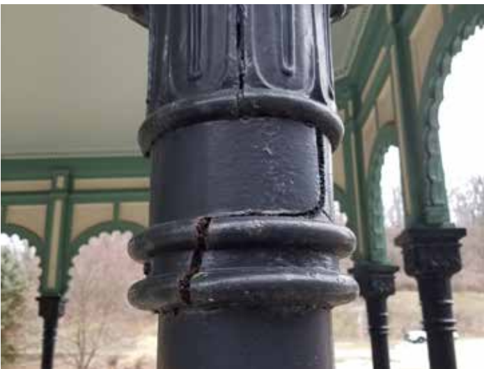
11. Cracked post at Eden Park
