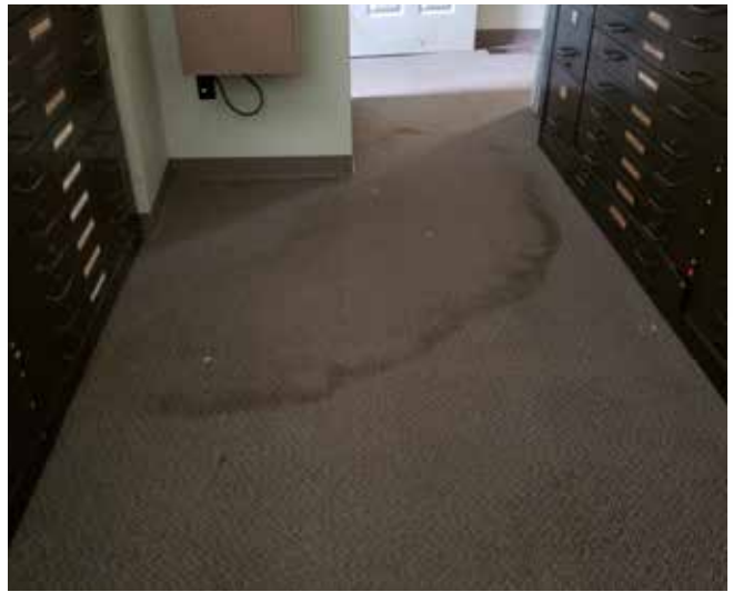
20. Planning Office wet carpet damage
