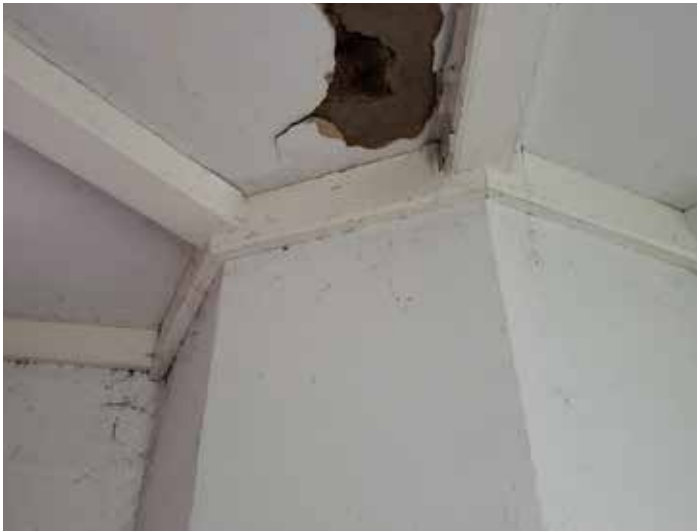
15. Seasongood Square CS interior damage
