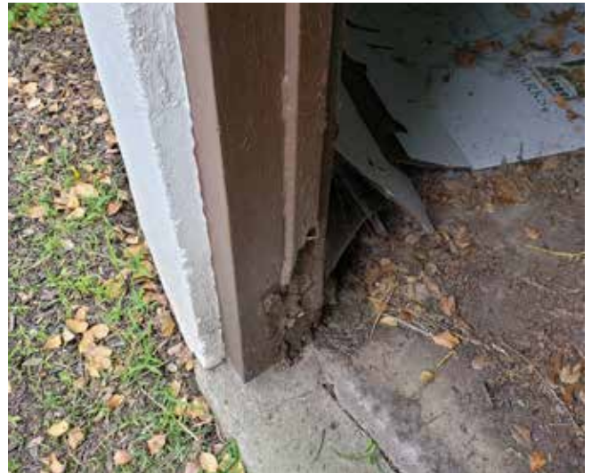
16. Seasongood Sq. CS rusted door frame
