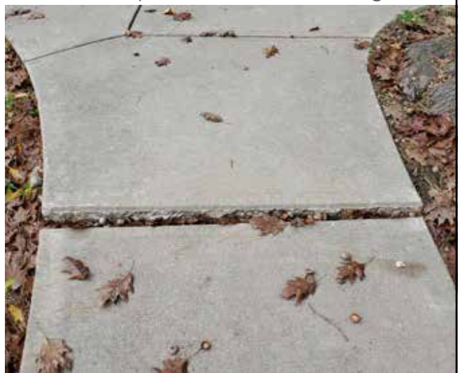
12. Kennedy Heights uneven sidewalk
