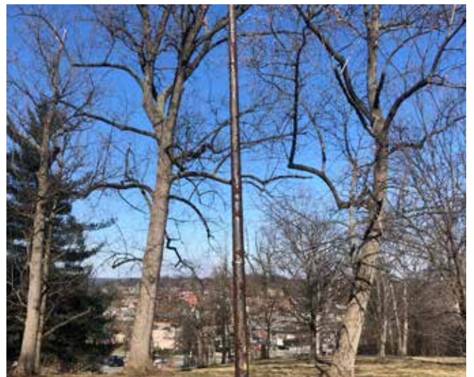
12. Rusted light post at Burnet Woods
