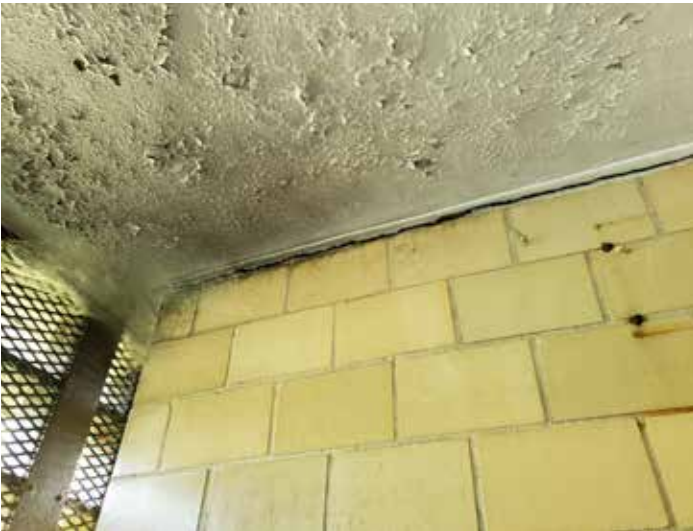
21. Mt. Echo CS ceiling damage
