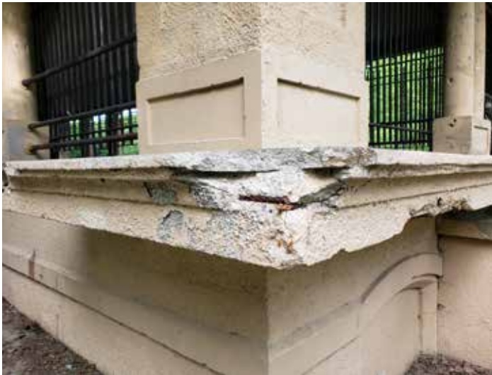
1. Inwood Pavilion decaying exterior
