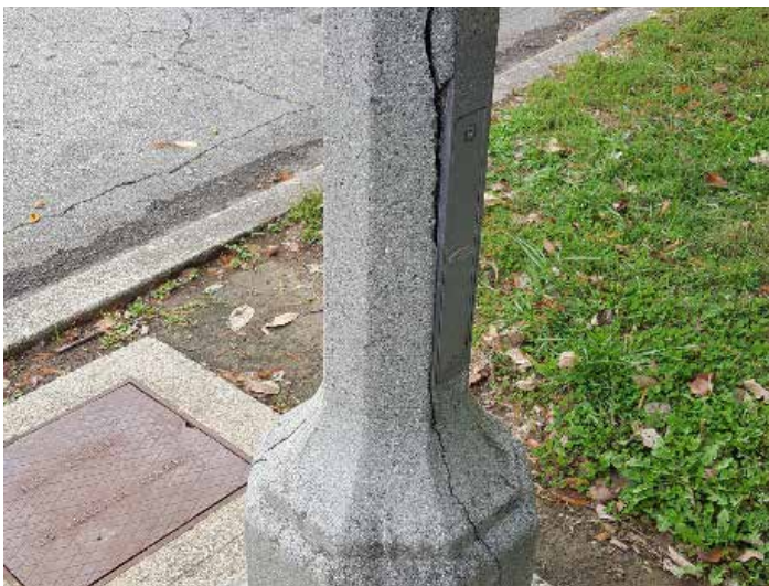
11. Cracked light post at Alms Park
