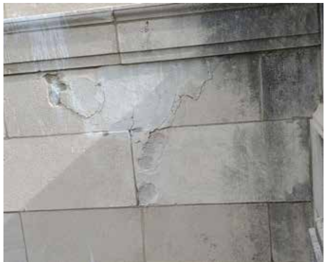
24. Ault Cascade delaminating sandstone
