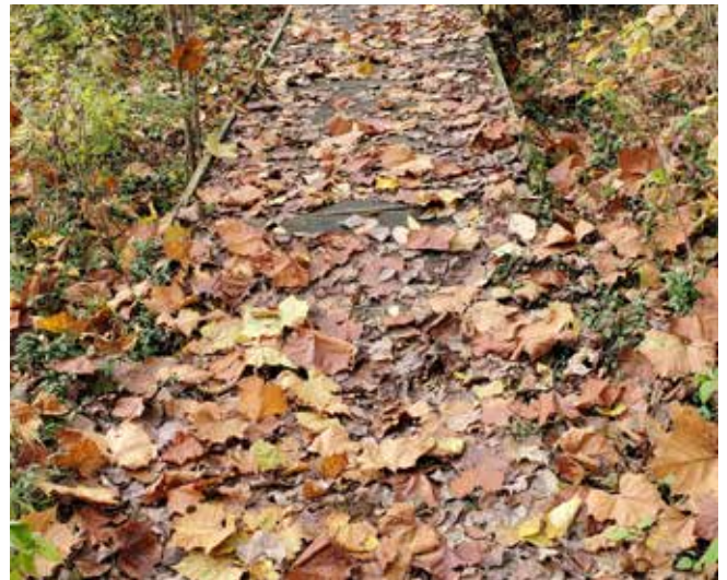
14. Kennedy Heights shaky footbridge
