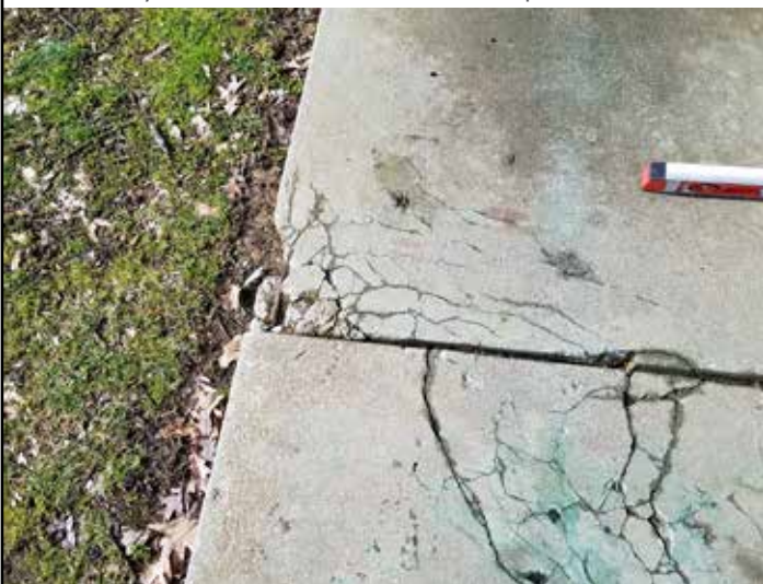
11. French Park cracked sidewalks
