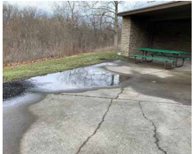
16. McEvoy cracked concrete
