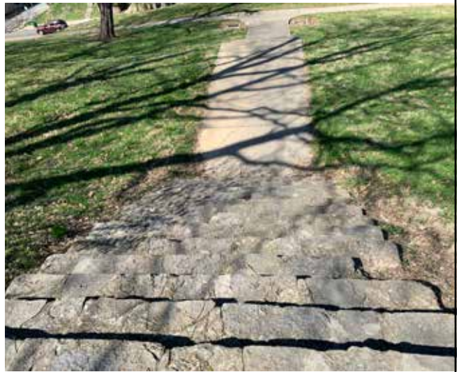
10. Glenway Park stairs with no railing
