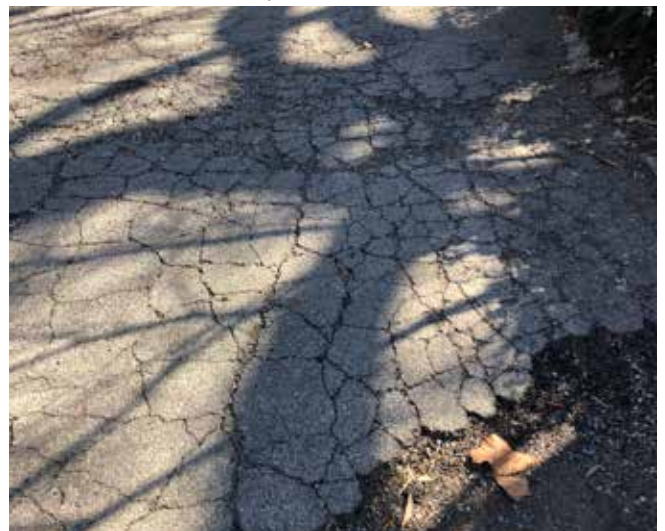
6. Hauck Gardens deteriorated pavement
