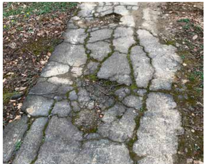
18. Arboretum damaged sidewalk
