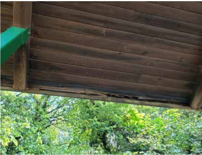
19. Fairview Shelter roof damage
