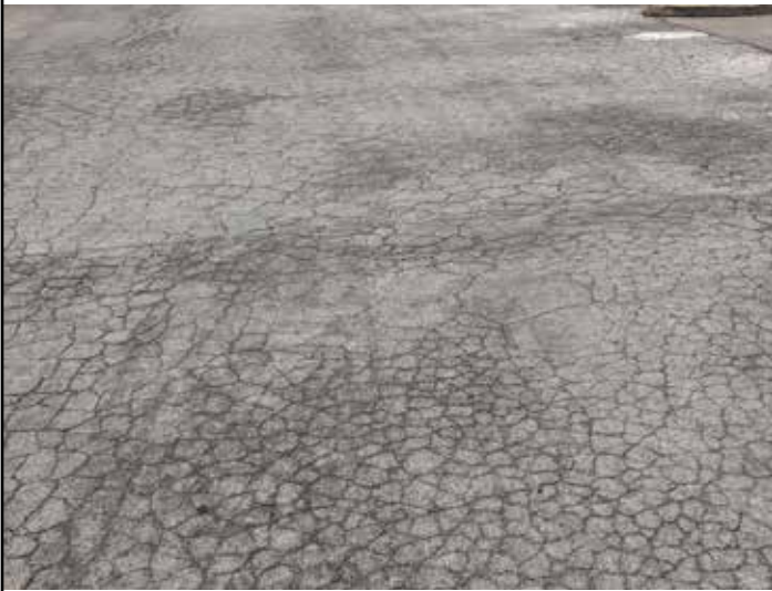
9. Sawyer Point deteriorated asphalt
