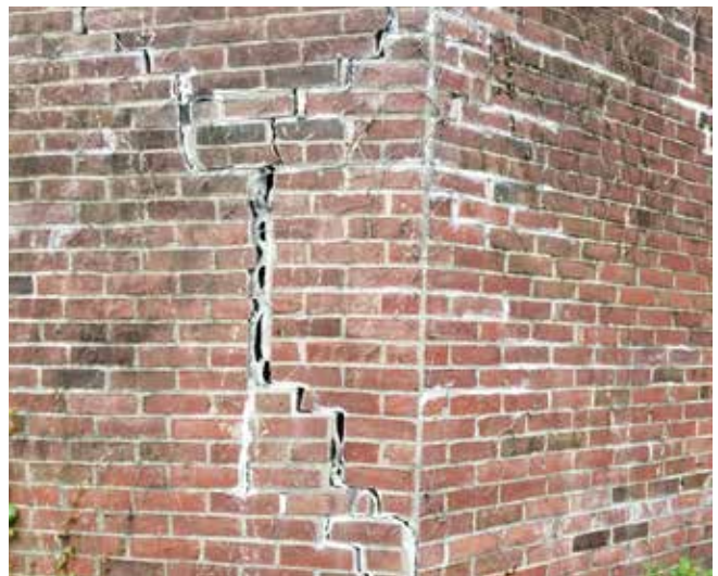
12. Cracked walls at Eden HQ Building
