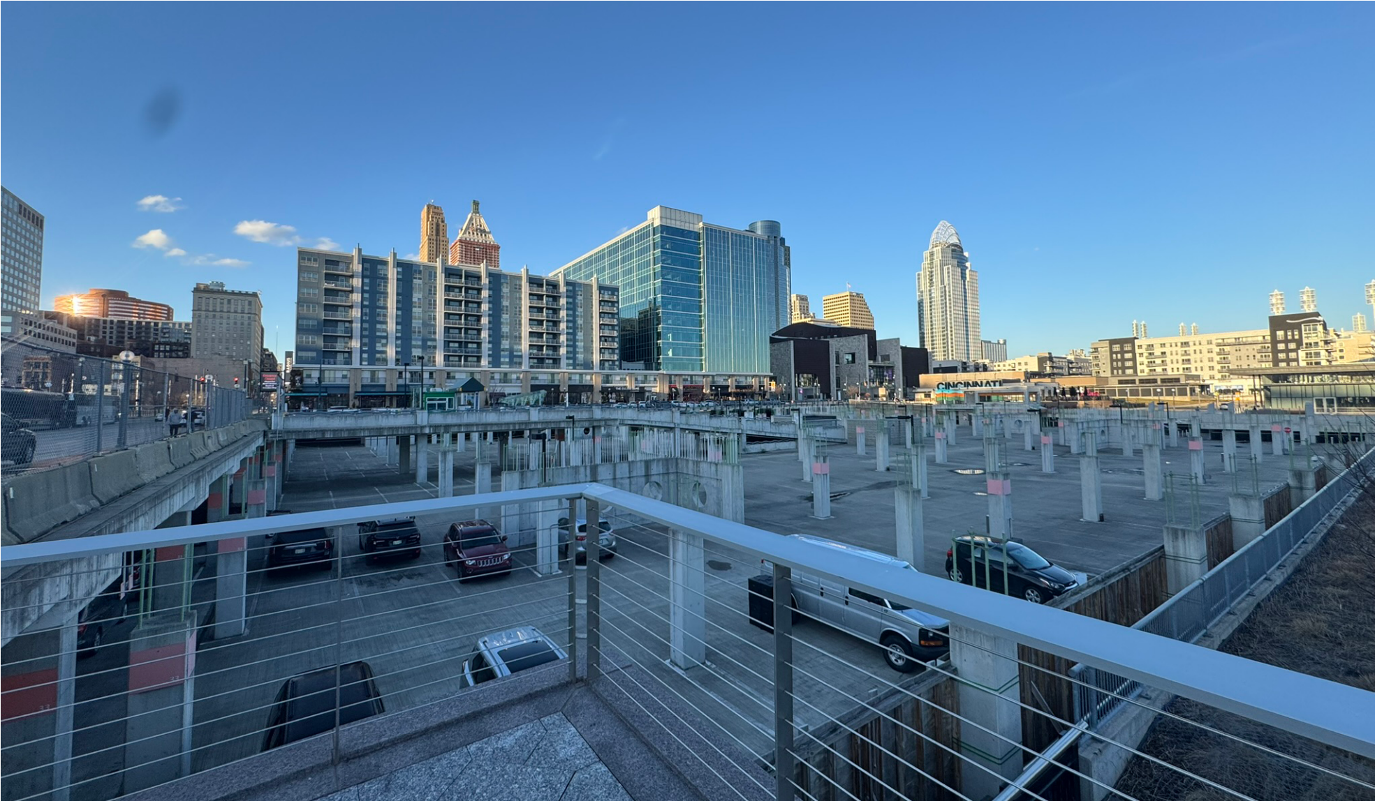
Images showing the existing structure built on Lot 24, south corner looking northeast.
