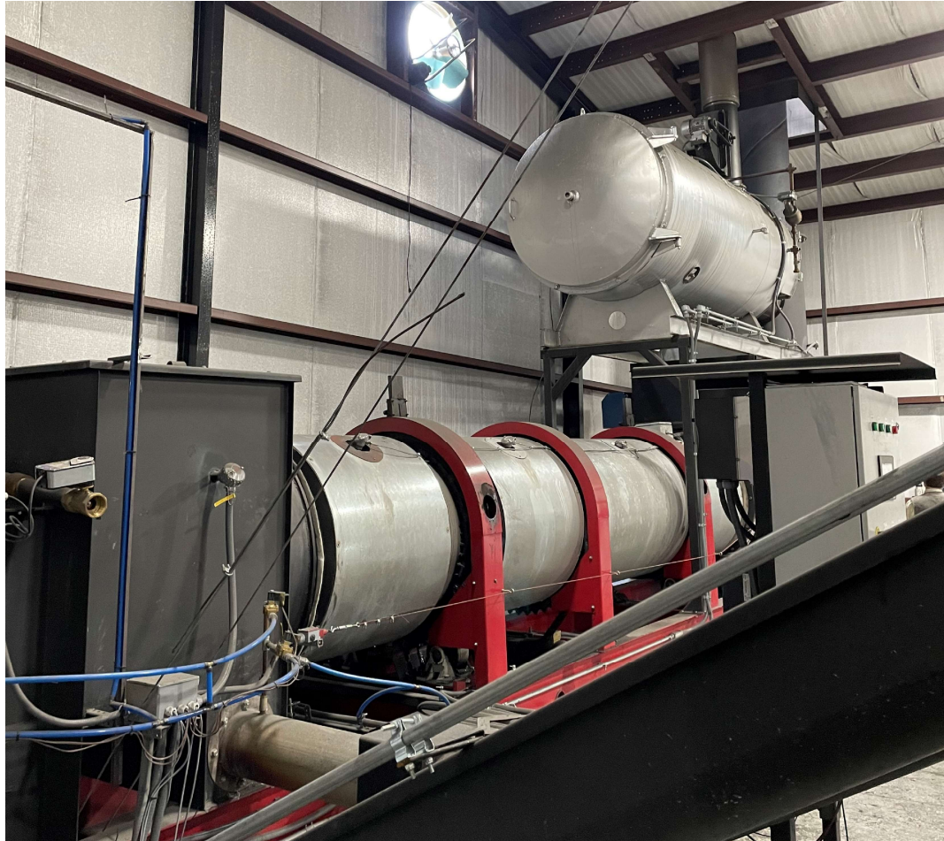
Boiler on top of Pyrolysis Unit
