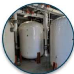
Thermal Energy Storage
