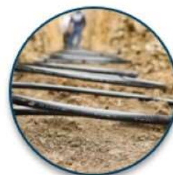
Ground Source Heat Pumps
