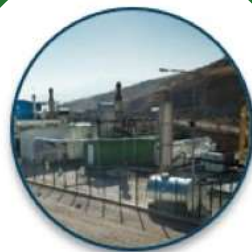
Combined Heat & Power
