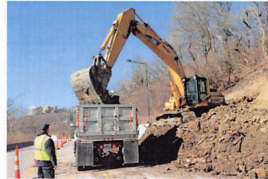
Cleanup of a landslide onto Columbia Parkway. Photo courtesy of City Staff.
