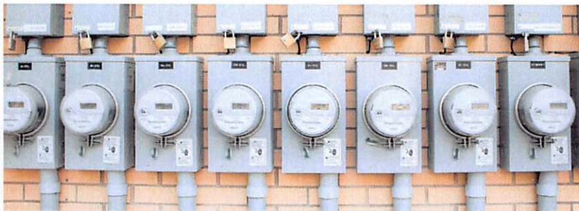
Electric meters on a multi-family building.
