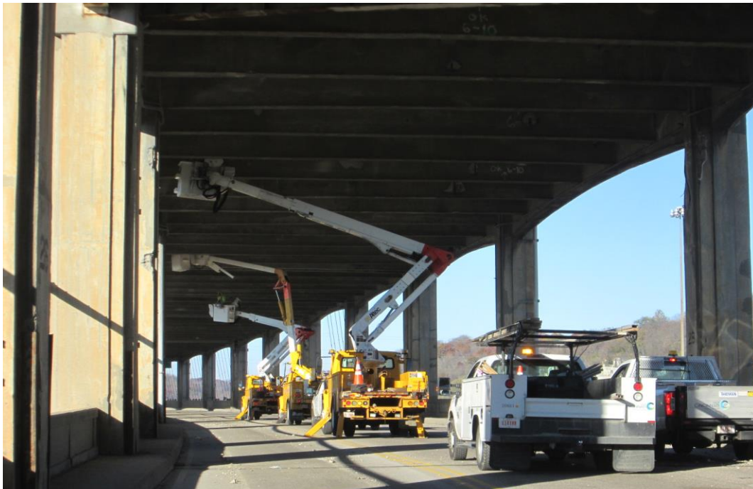
Removal of loose concrete from the Western Hills Viaduct as part of the biannual routine maintenance.
