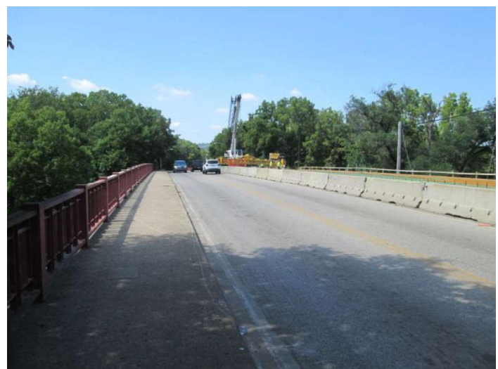
Ongoing part-width construction work at the Galbraith Ave Bridge over Anthony Wayne and RR
