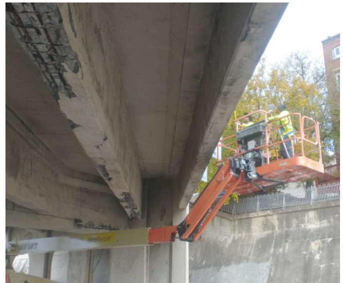
Removal of delaminated concrete from the Brighton Street Bridge over Central Parkway.
