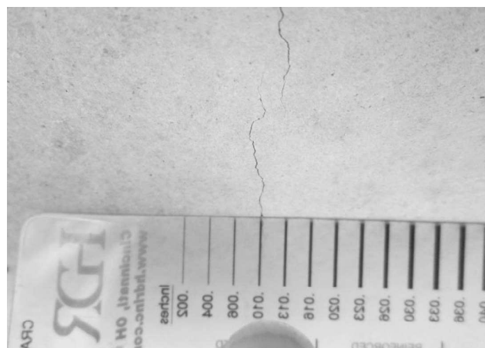
Above: monitoring cracking in prestressed concrete box beams, here van Hart bridge over Lick Run
