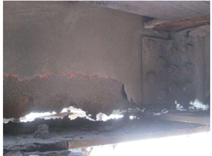
Above: Perforated floorbeams under the Gest Street Chessie overhead – 1 st East of the Mill Creek.
