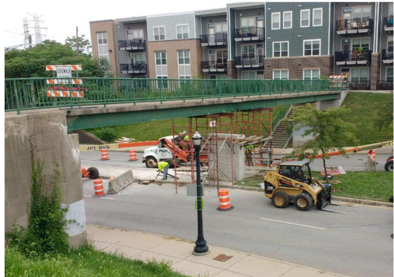
Madison Road Pedestrian overpass west of IORY, during construction (above 2020) and after completion (below 2021)
