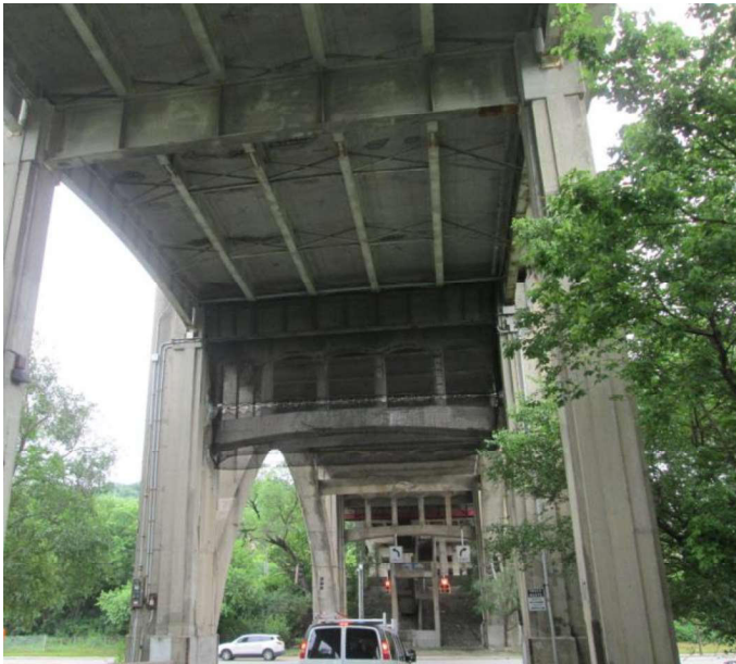
Debris netting under the Western Hills Viaduct west of Spring Grove Avenue
