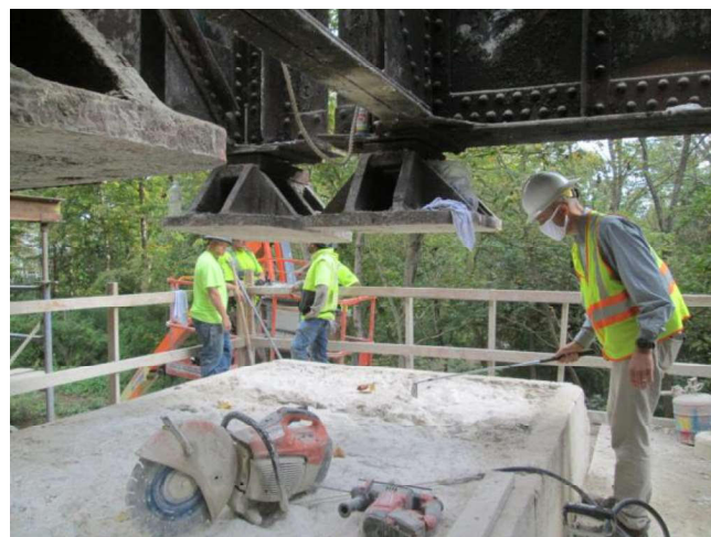
Above: 2021 Pier cap reconstruction at the Wasson Way Bridge over Ault Park.
