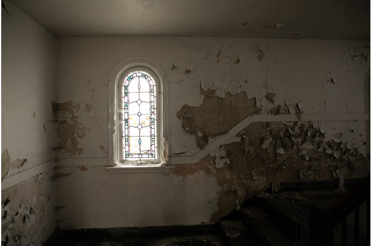
Figure 10 View of stair hall with arched, leaded glass window. Walls exhibit paint failure and plaster damage.
