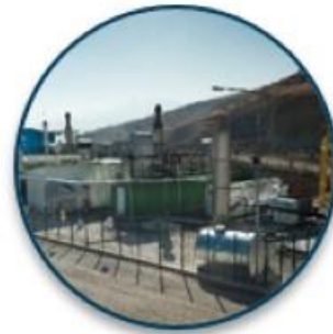
Combined Heat & Power
