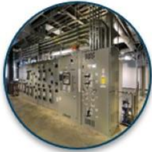
Battery Energy Storage
