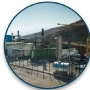
Combined Heat & Power
