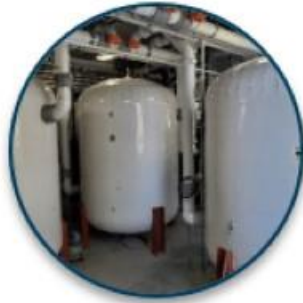
Thermal Energy Storage
