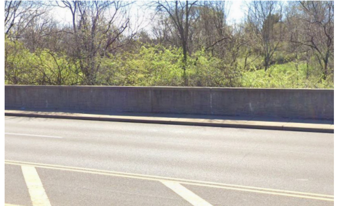
Current sidewalk conditions between Hawaiian Terrace and Shepherd Creek Road along Colerain Avenue
