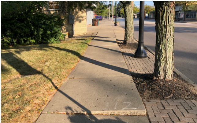
Current sidewalk conditions in the Mt. Airy NBD in the 5500 Block of Colerain Avenue
