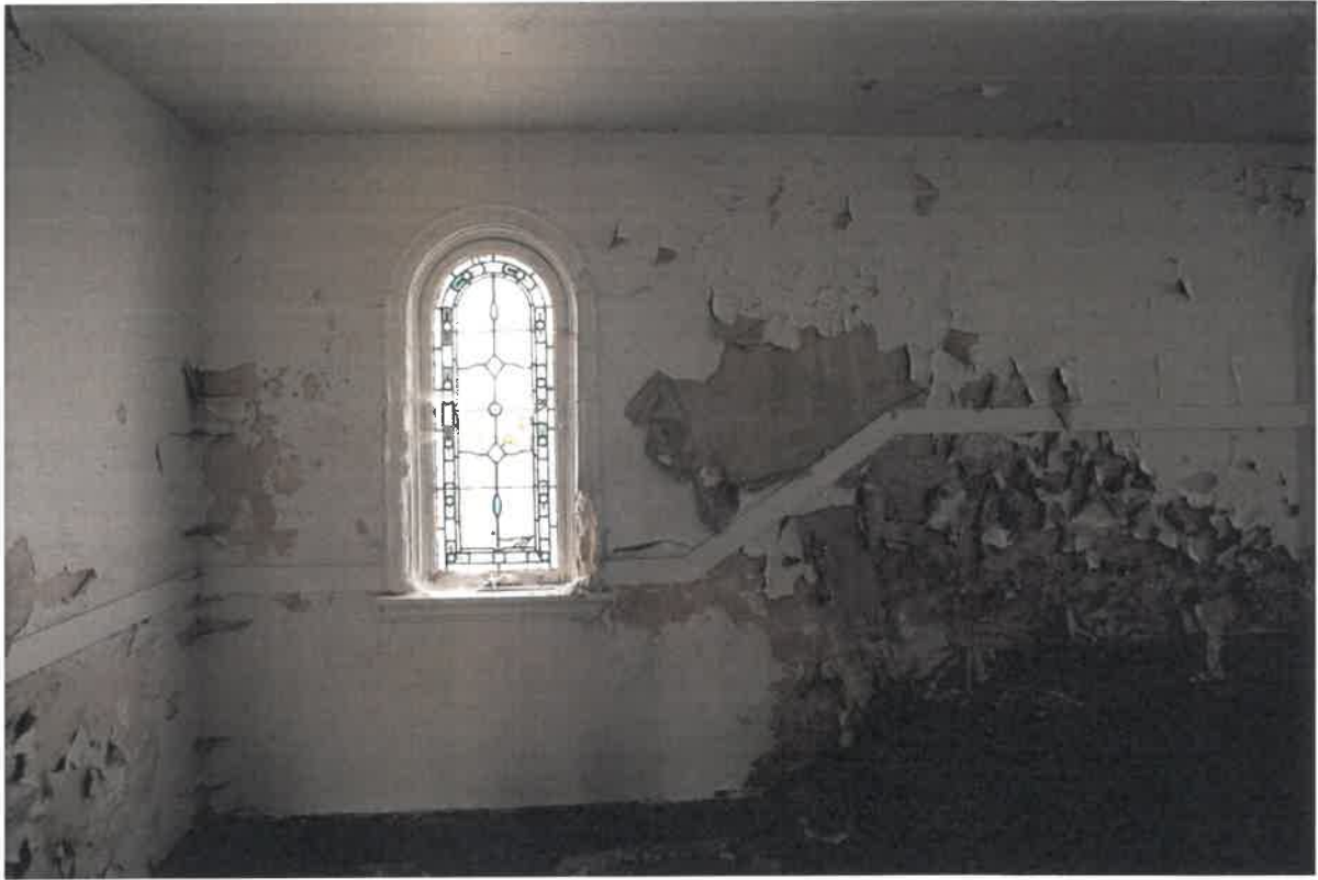
Figure 10 View of stair hall with arched, leaded glass window. Walls exhibit paint failure and plaster damage.
